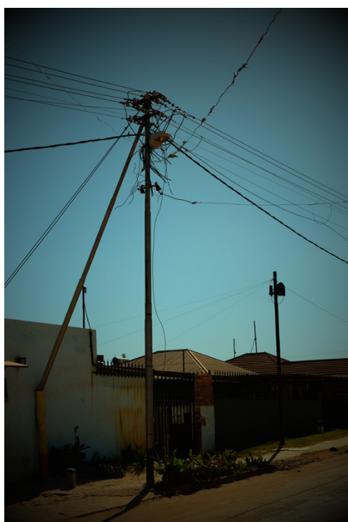
Illegal electricity connections, Johannesburg, June 2026. Photo supplied
